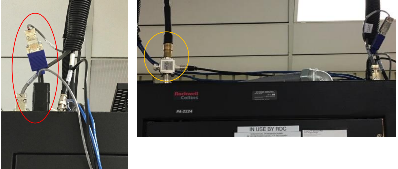
Figure B-5. Transmitter antenna interlock circled in red (left) and installed RF tap circled in orange (right).
