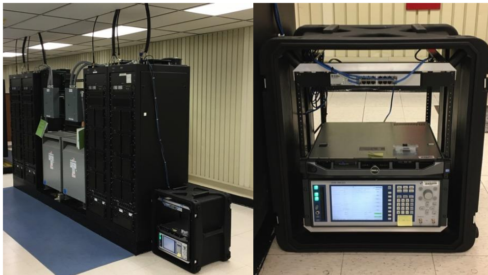
Figure B-2. (Left) Kodiak HF transmitter #12 (tall cabinet on end) and portable server rack, (Right) close up of the portable server rack housing the content server, DMOD3 modulator, and Ethernet switch.
