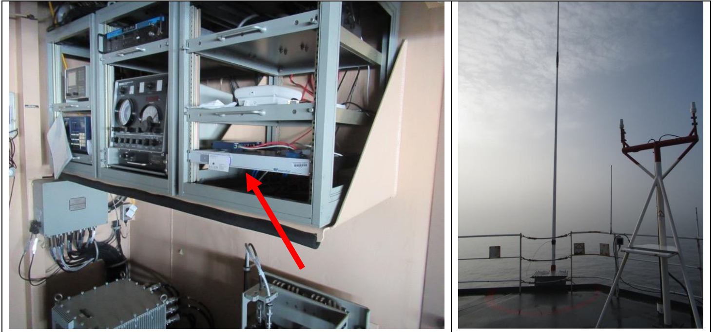
Figure B-13. DRM receiver installed in USCGC HEALY's radio room. The antenna on the port side flying bridge was used.
