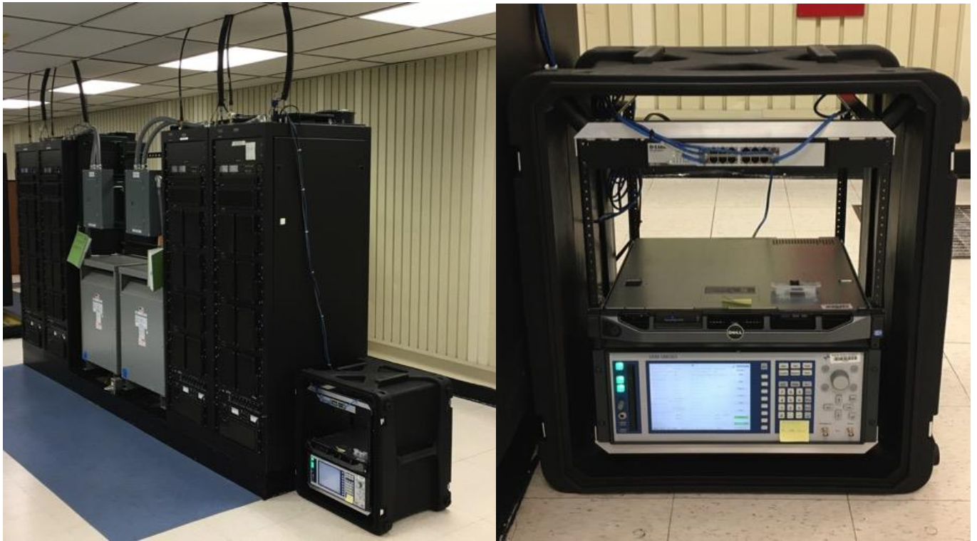
Figure 5. (Left) Kodiak HF transmitter #12 (tall cabinet on end of row closest to viewer) and portable server rack. (Right) Close-up of the portable server rack housing the content server, DMOD3 modulator, and Ethernet switch.
