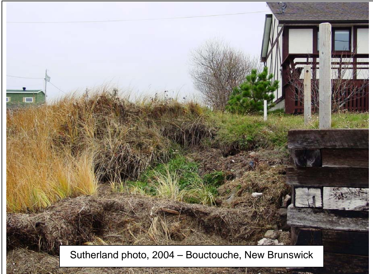
FIGURE 6.10 – POORLY CONSTRUCTED EROSION CONTROL STRUCTURE
